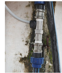
Water flow meter
